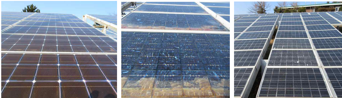
Fig. 5 Example of PV Damage, yellow, Wet, Crack
